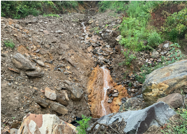
Before and after: culvert conditions following Hurricane Helene, showing recovery and plant regrowth.
